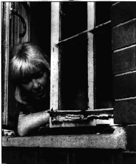
● HOPES DAMPENED - headteacher Wendy Smith says school corridors leak in half a dozen places, and in classrooms displays of work and books are ruined
